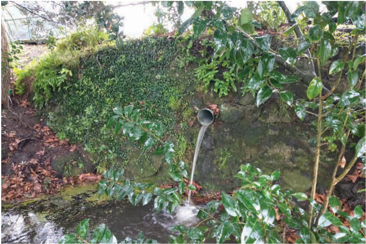
Figure 15. Dam and culvert on southern side of Farm Road in vicinity of new stormwater trenching.
